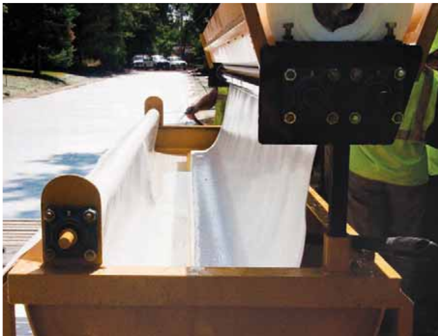
The contractor fabricated an efficient moving platform to place a wet-curing membrane over the freshly placed pavement. PHOTOS: JOE NASVIK
