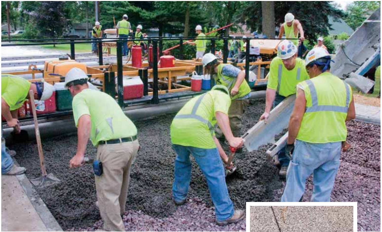
Two ready-mix trucks backed up side by side in front of the roller screed to place concrete in the 21-ft.-wide street. Concrete flowed freely down the chutes and new trucks arrived every 25 minutes. PHOTO: JOE NASVIK
