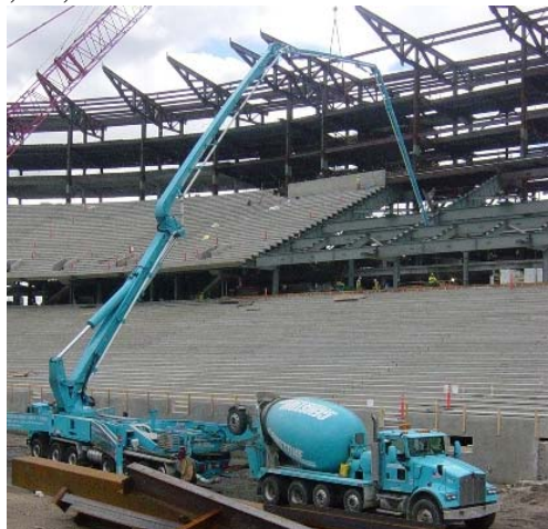
Cemstone’s Kenworth trucks are helping build the University of Minnesota’s new football stadium (above and at right).
